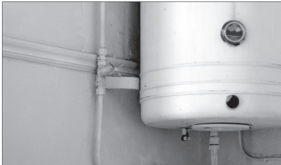
When using a hot water heater – part of the Combustion Appliance Zone – it's important to make sure it's in an area that is well ventilated.
