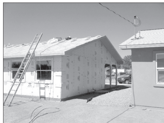
The Otero County Habitat for Humanity used rigid insulation installed at the exterior walls of a home, which was built to Build Green New Mexico silver certification in Tularosa.
