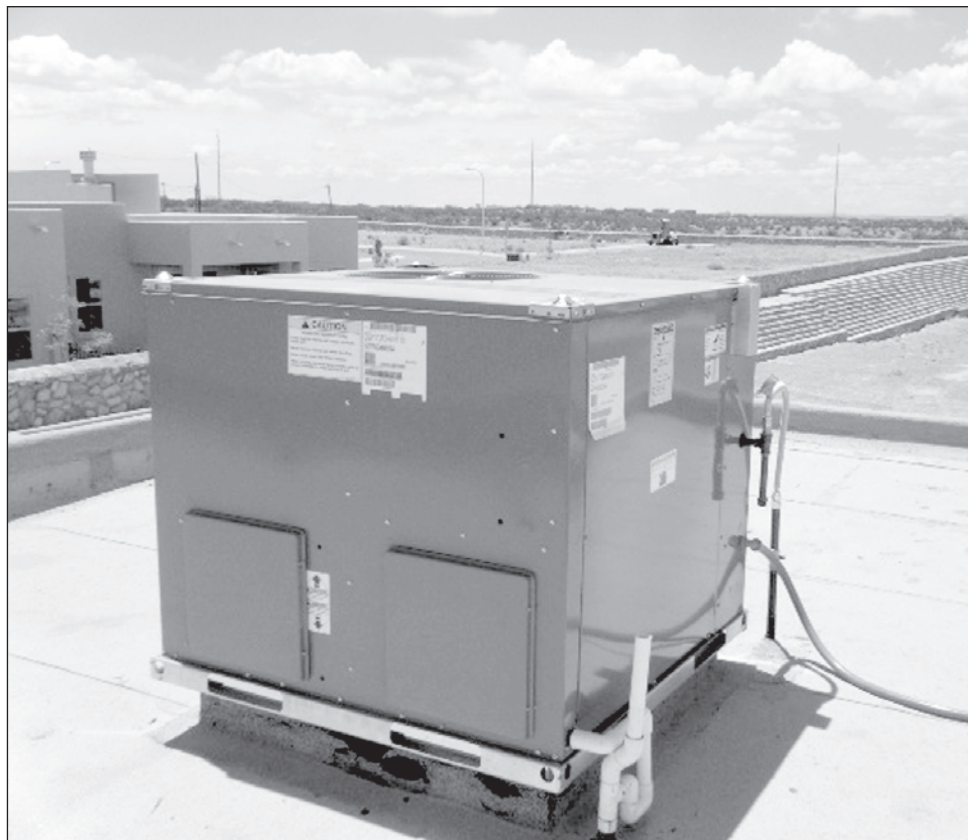
Stay cool this summer by properly maintaining your rooftop mounted package air conditioner and gas heating unit.
