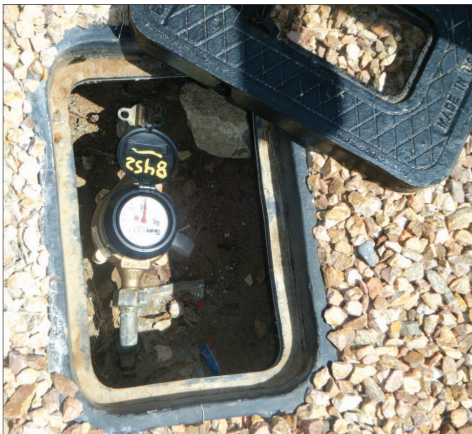
A quick check at your meter dial will let you know if you have unseen leaks on your property.
