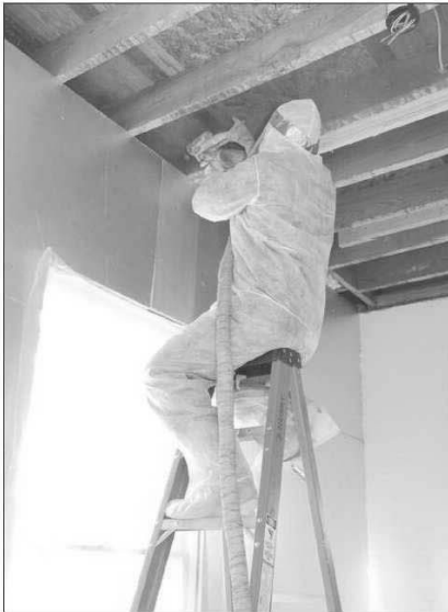
A McGinley Construction worker blows expanding foam insulation into the wall of this proposed Green Build New Mexico home built in 1908 near Pioneer Park. The foam will help provide better insulation.
